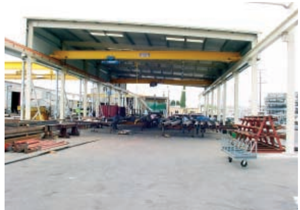
Free-Standing Covered Craneway
