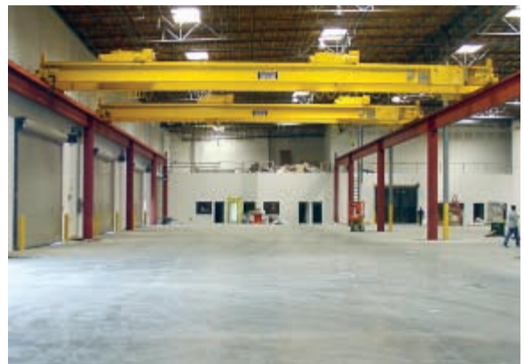
10-Ton Top Riding Cranes & Runway
