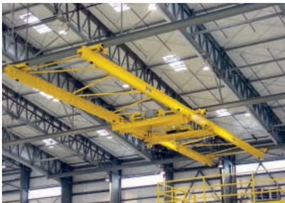
20-Ton Underhung Crane System
